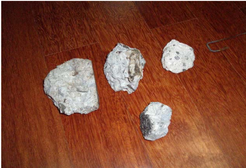
Figure 4: Broken pieces of concrete found on the runway.
